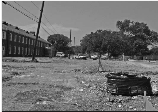
Work continues on the church's new parking lot, which is expected to be completed by the end of the month. (above)
